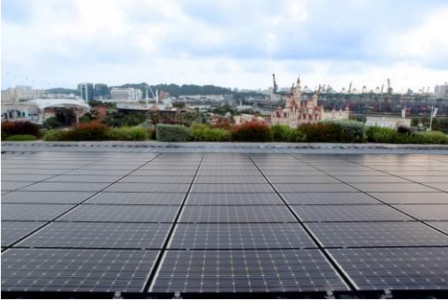
One of Singapore's largest solar photovoltaic installations at Resorts World Sentosa
